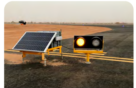
Solar LED ERGL in position to signal entry onto active runway.
