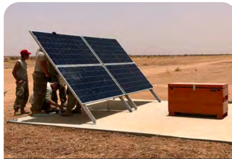
The entire solar airfield lighting solution, including these solar panels and battery boxes, were installed in less than two weeks.
